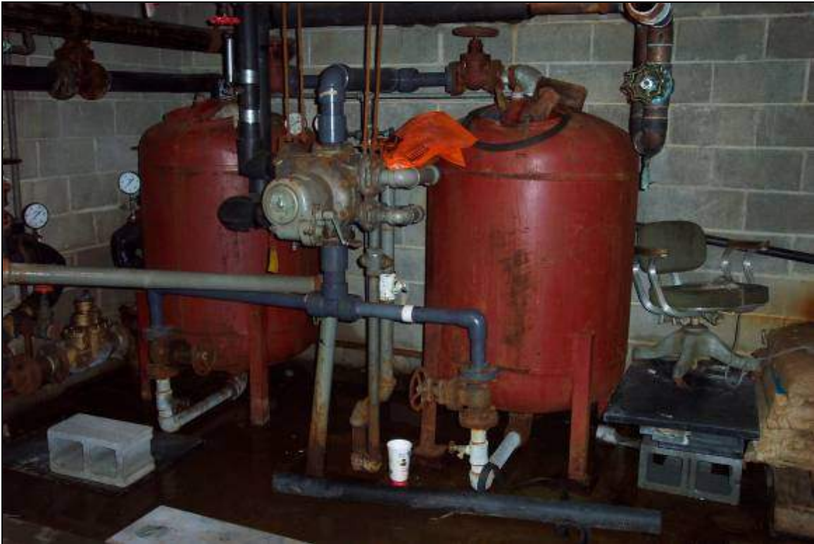
View of water filter system located in the basement of Building A. Water was visible beneath the filters due to ruptured pipes.
