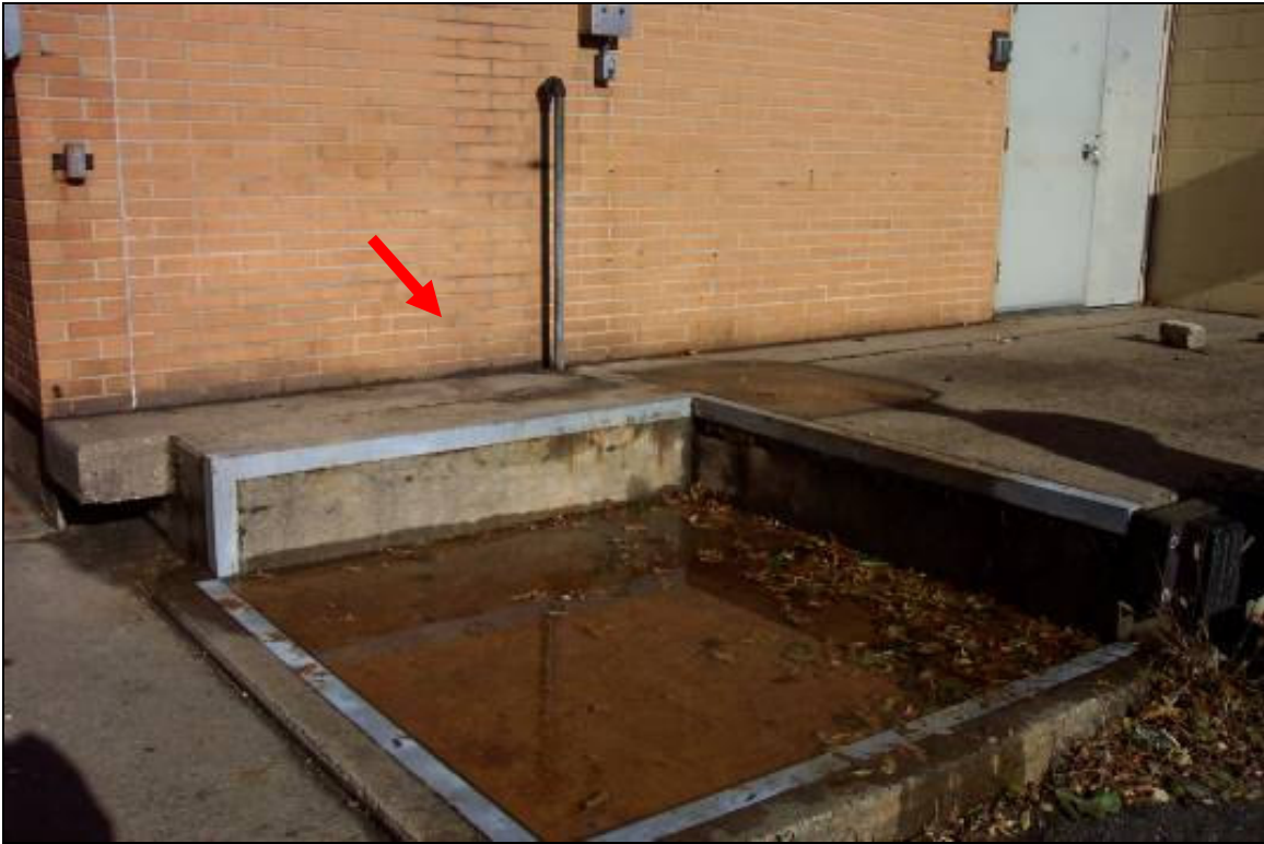
View of the former location of above ground hydraulic oil tank and former lift located at the dock of Building B
