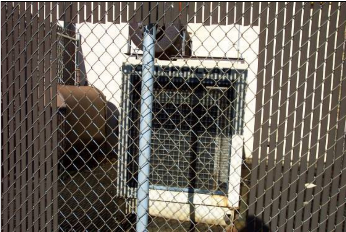
View of emergency generator associated with the 275-gallon AST located at south exterior of Building B
