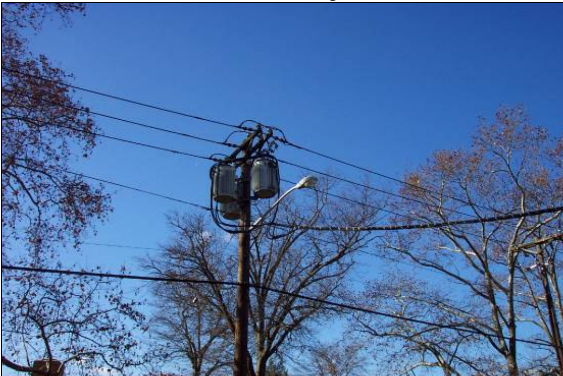
View of pole mounted electric transformer located along Davis Street adjacent to Camden Laboratories. No leaking or staining observed.
