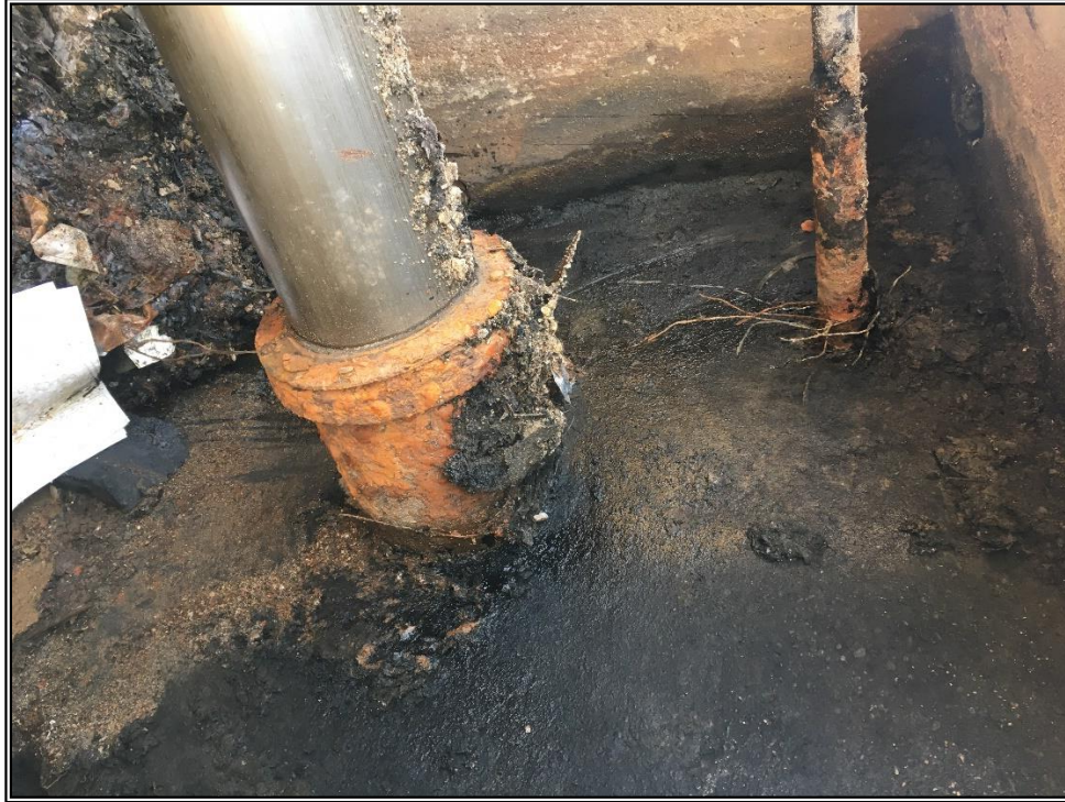
Photo 7: Hyrdaulic Pit (Interior)
