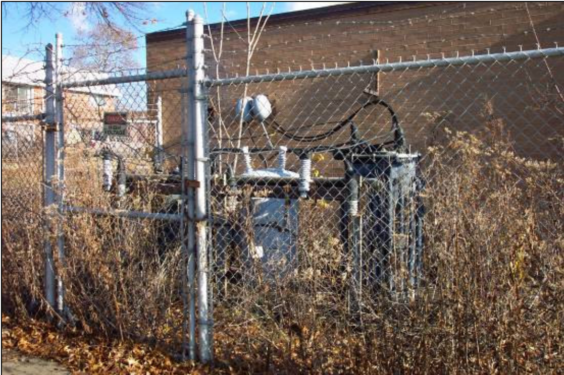
View of electric transformers located adjacent to the west of Building D. Staining could not be determined due to overgrown vegetation.
