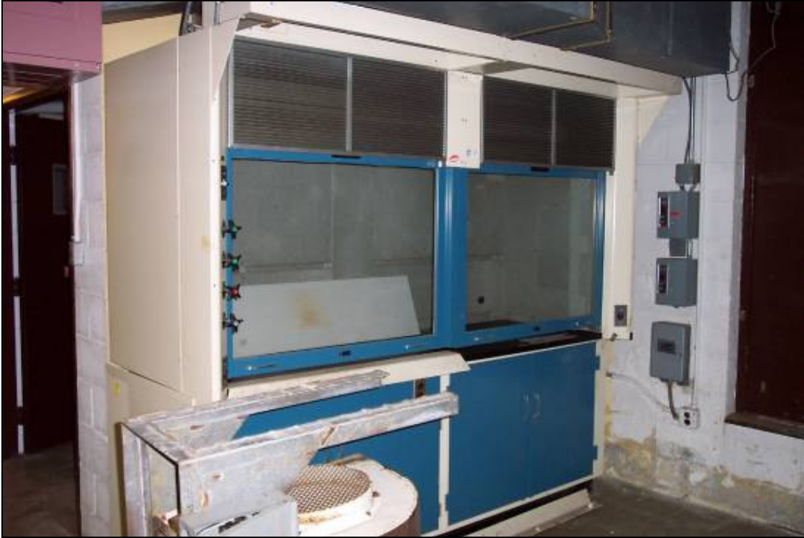
View of laboratory vent hood located in the ground floor of Building F
