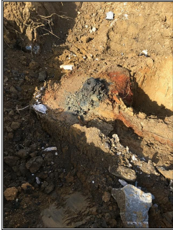
Photo 9: Hydraulic Pit – Soil Staining
