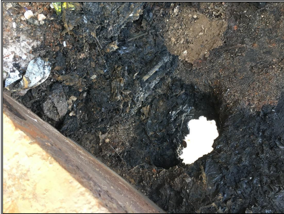
Photo 8: Hydraulic Pit Hole
