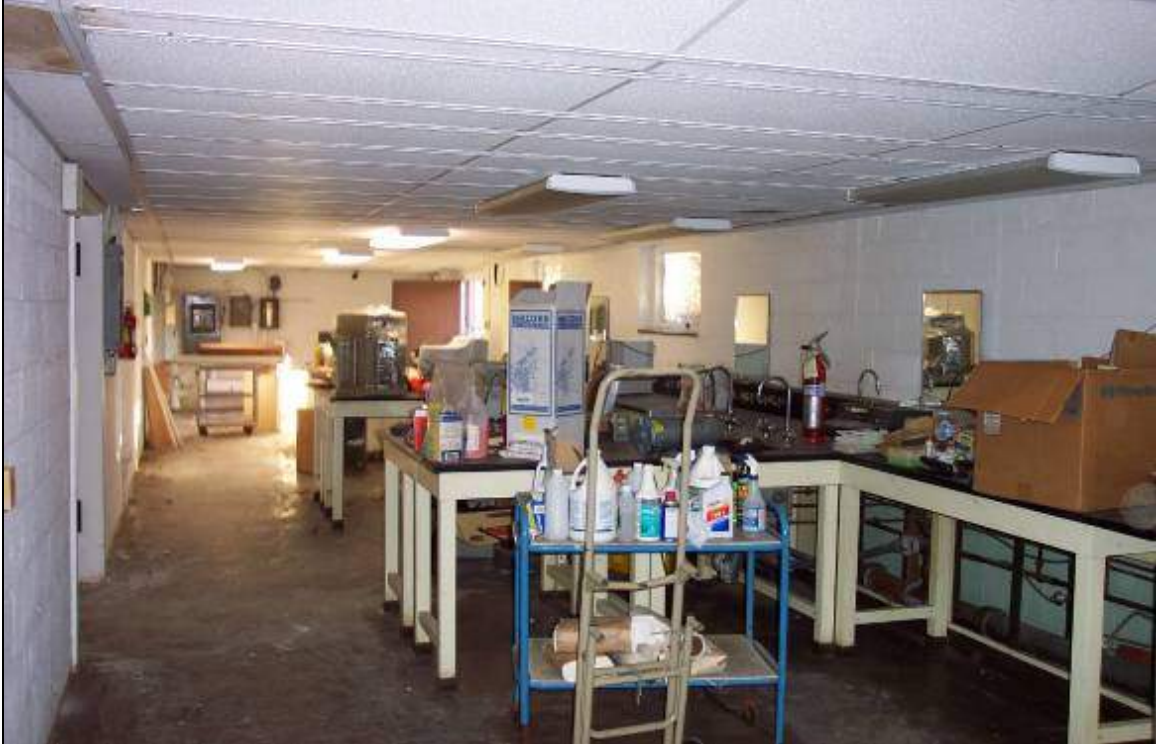
View of cleaning supplies located in the first floor laboratories of Building A. No leaking or staining observed.
