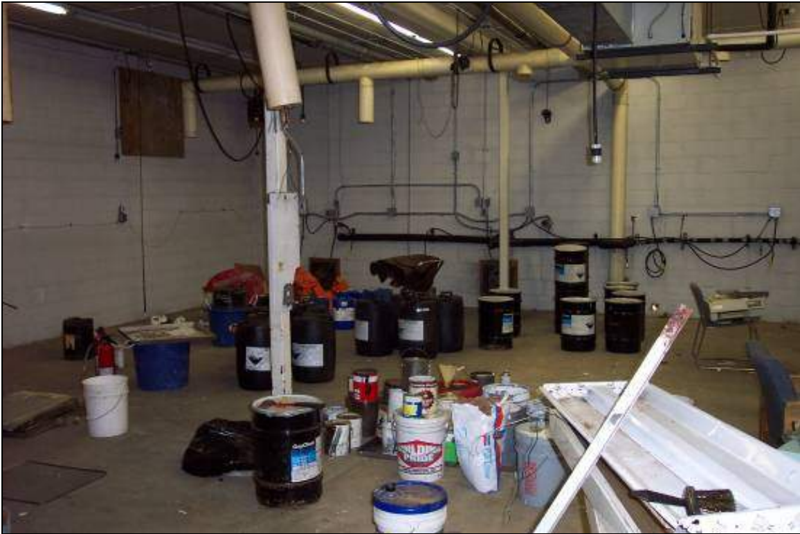
View of freezer room of Building B. Four (4) containers of muriatic acid, five (5) containers of caustic soda and several empty five (5) gallon containers were noted. No staining was observed.
