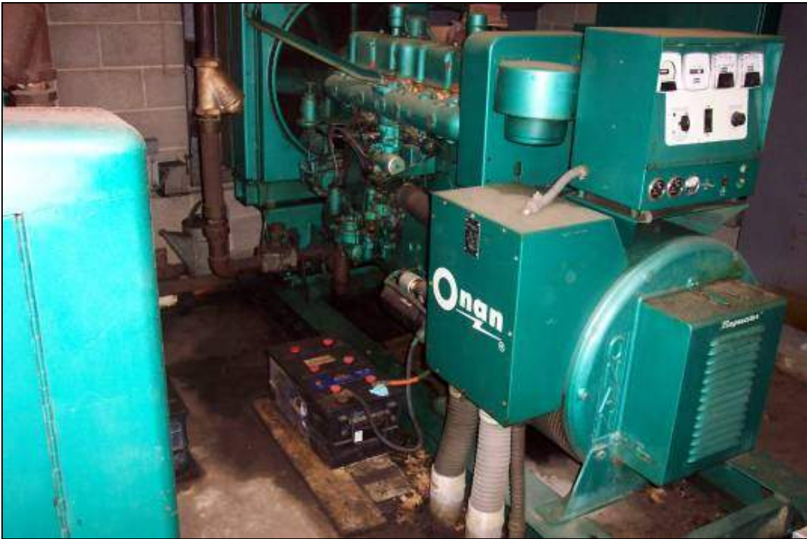
View of emergency generators located in Building D. Staining observed beneath the generators.
