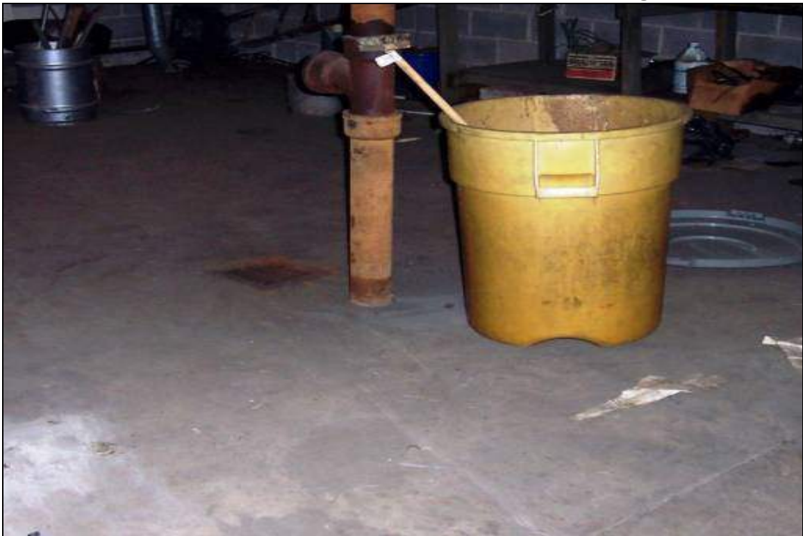
View of boiler room in Building B. No staining noted in the area of the floor drain.
