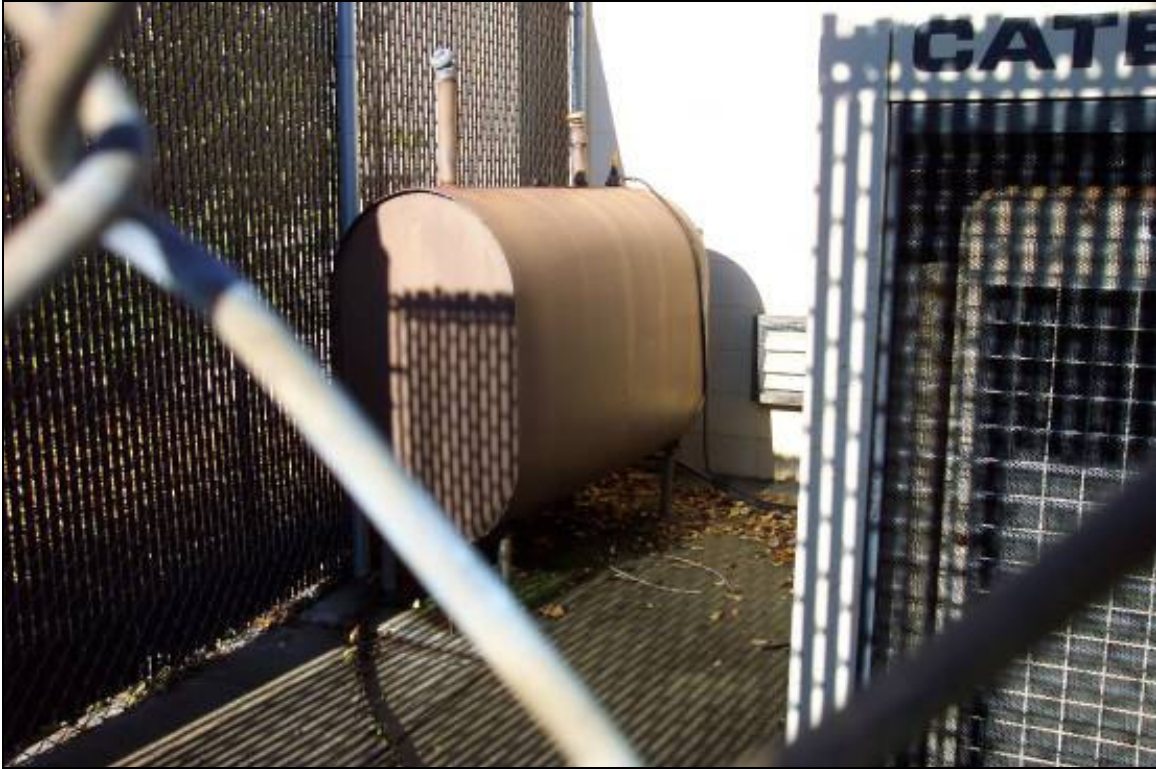
View of empty 275-gallon AST formerly containing diesel fuel located at south exterior of Building B. No staining noted.
