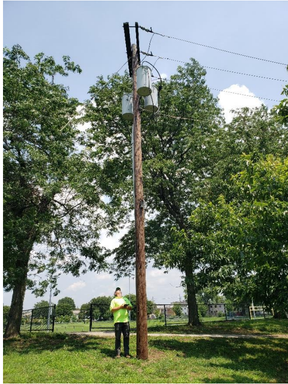
Photo-11: View of AOC-5: Pole Mounted Transformer.
